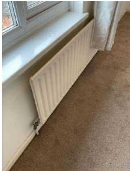
Single panel radiator
