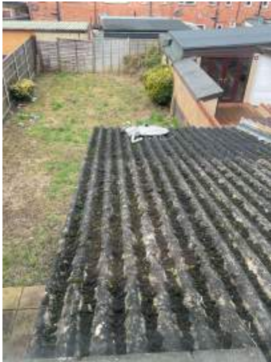
Possible, asbestos corrugated roof
