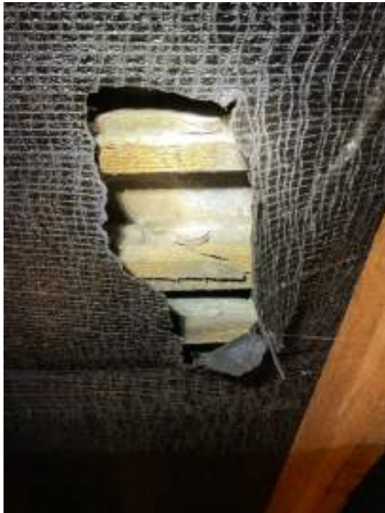
Battens cracked and torn felt
