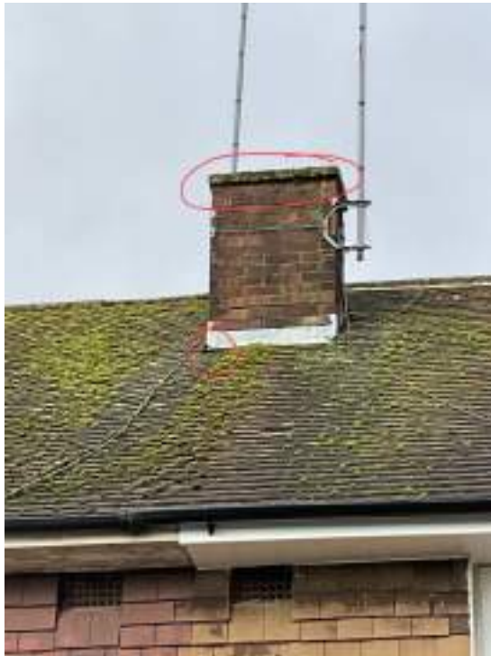
Minor defects noted
