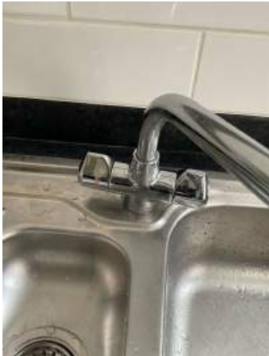
Loose tap fitting
