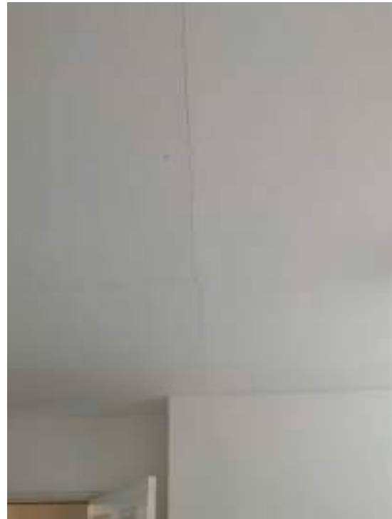
Hairline thermal cracks
