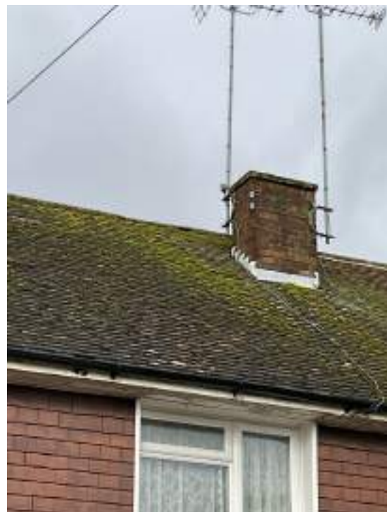
Ridge tiles loose neighbouring property
