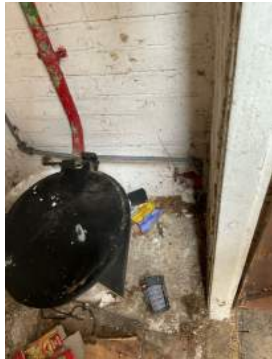
Stop cock to outbuilding
