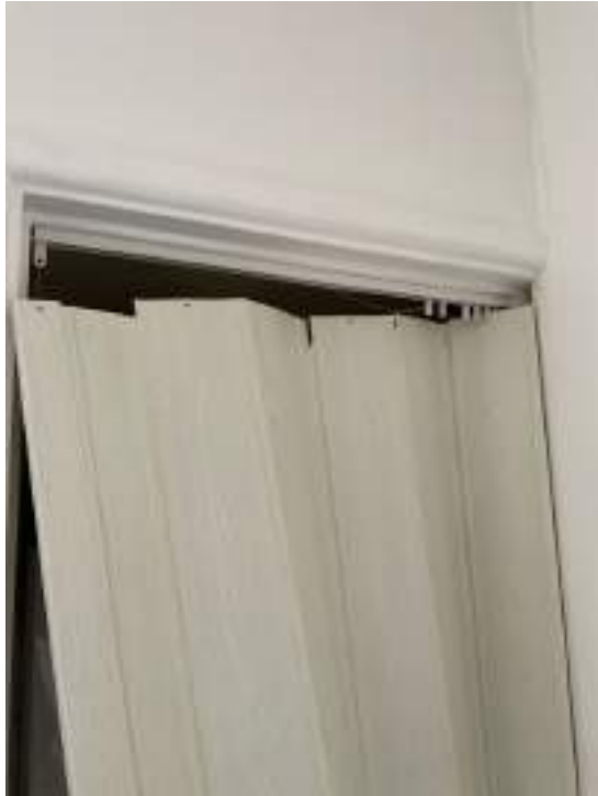
Door screen to boiler broken
