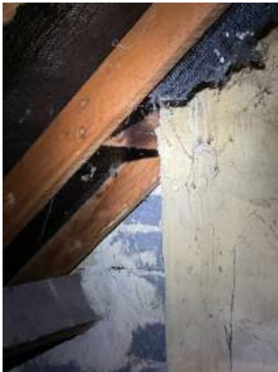
Slight rot to timbers
