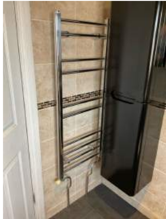
Heating to bathroom
