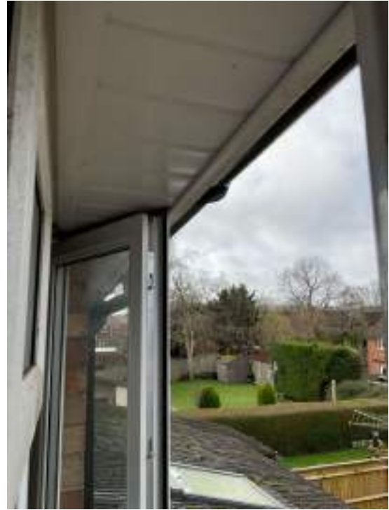
Windows on FF unable to open
