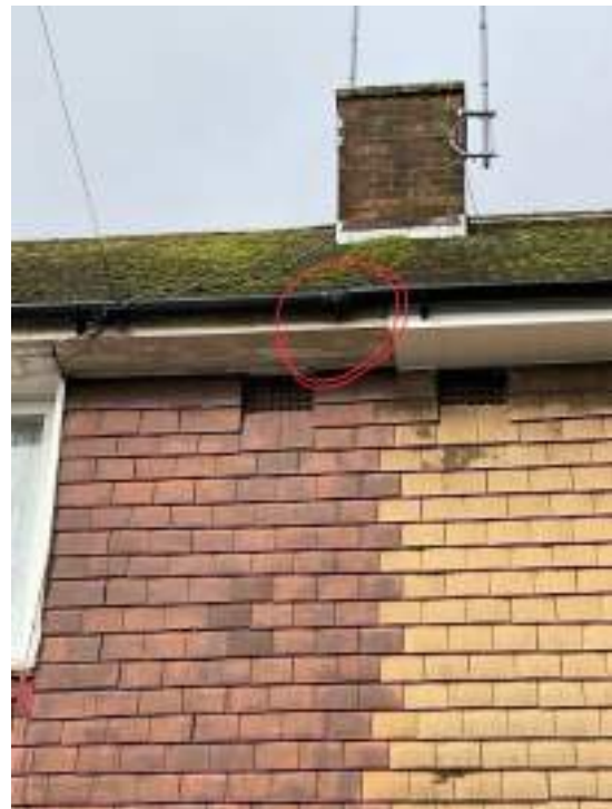
Leaking connection Front elevation
