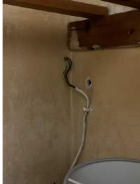
Wires in openings especially when required to be
