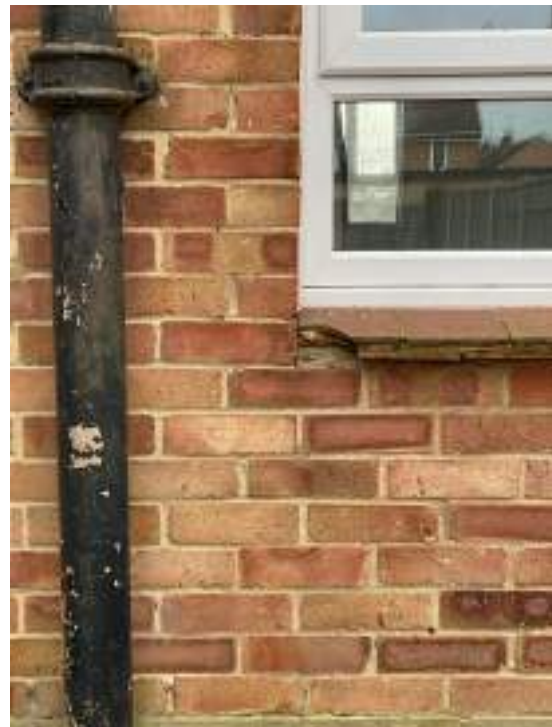
Damage to tiles
