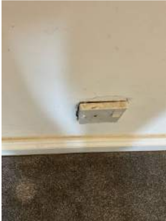
Loose fitted sockets
