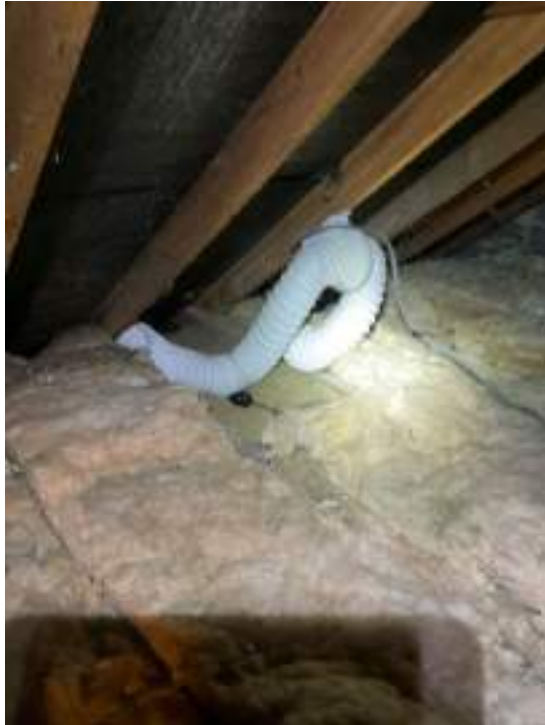
Tangled bathroom ducting
