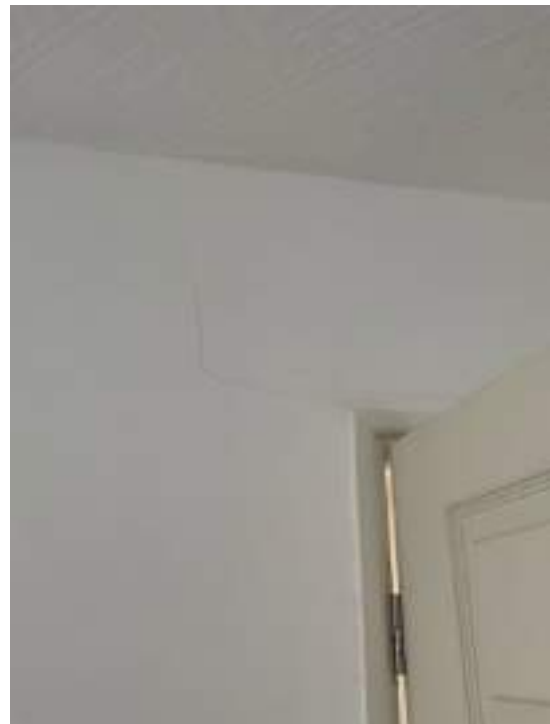
Hair line cracks
