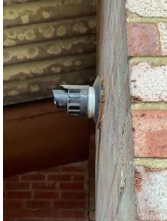
flue condition should be checked
