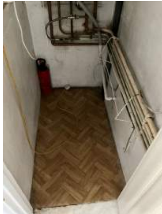
Damp readings in this area only
