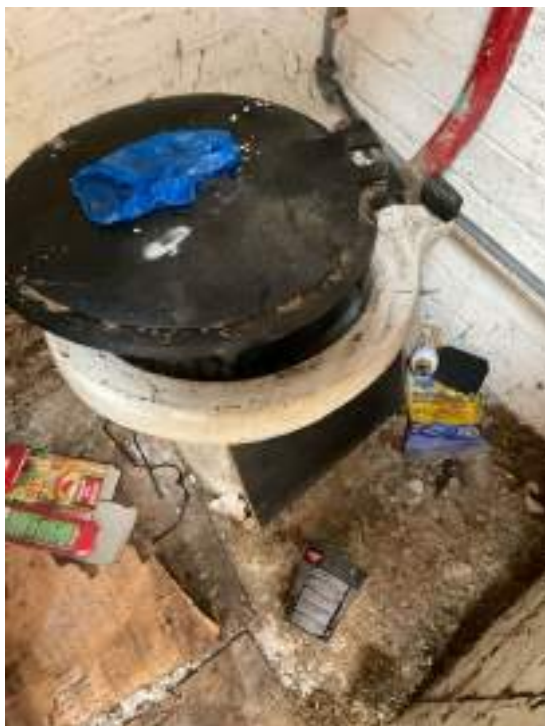
Possible asbestos toilet seat cover redundant
