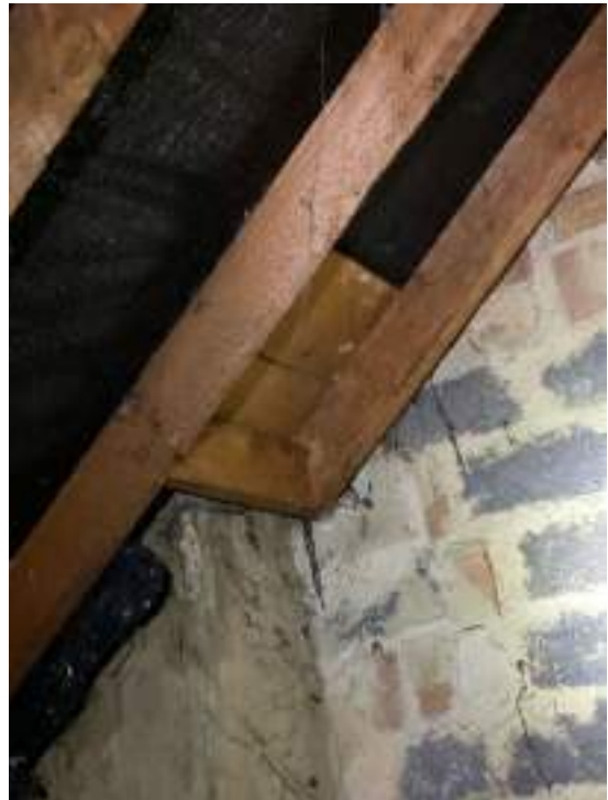
Breast in loft suspect area for leaks
