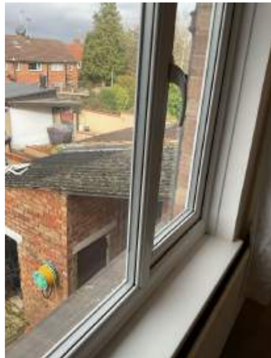
No installation date stamp on Windows
