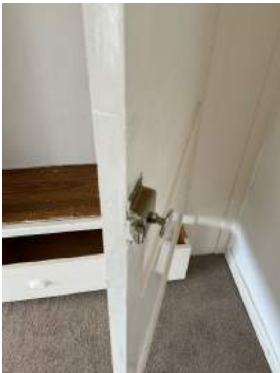
Bedroom cupboard lock handle broken
