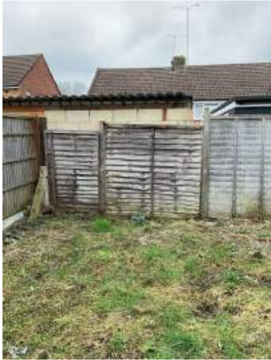
Fencing and garden needs to be replaced or redecorated
