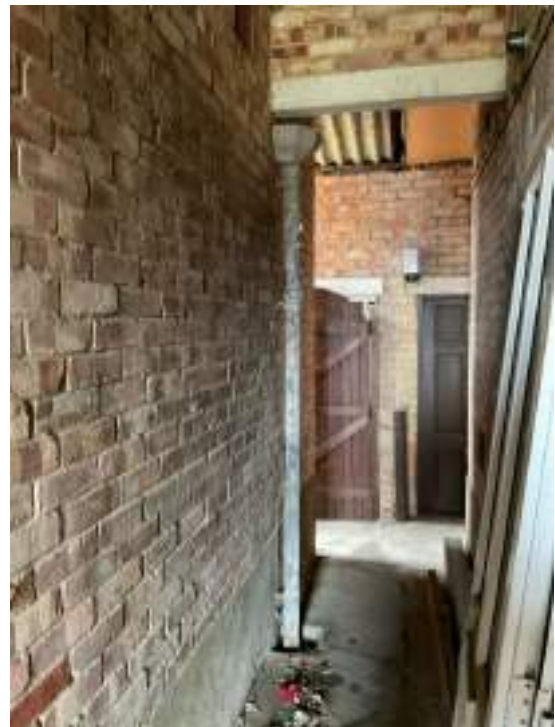
May contain asbestos fibres
