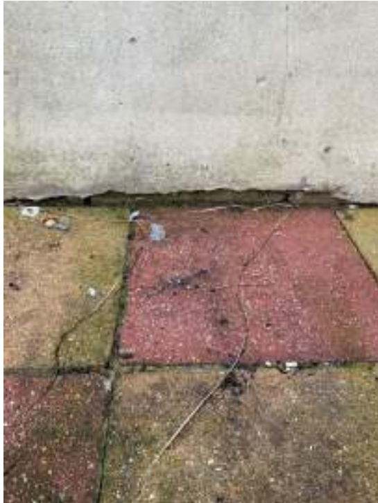
Cement plynth damaged this can leak in water repairs required
