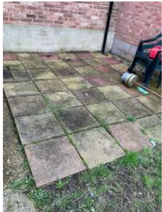
Various slabs, uneven
