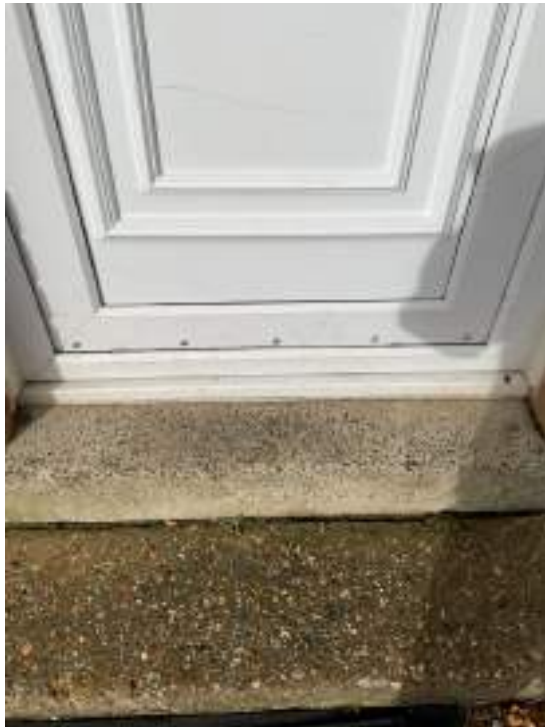
Weather guard missing
