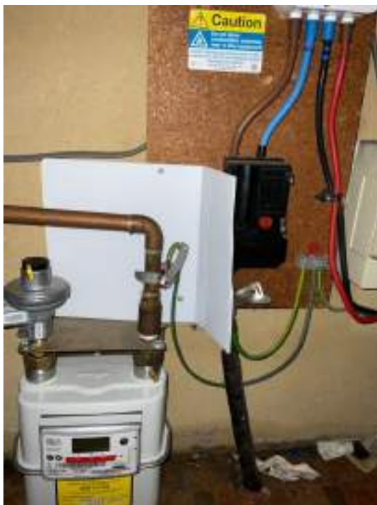
non conductive barrier
