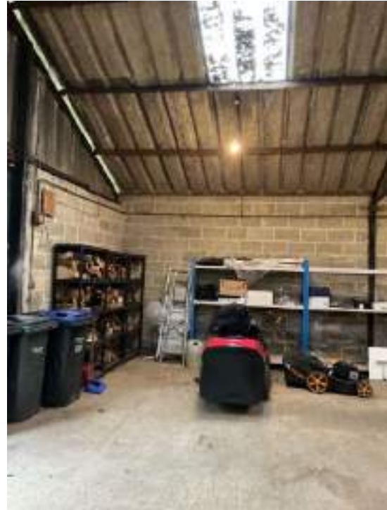
Possible asbestos containing material
