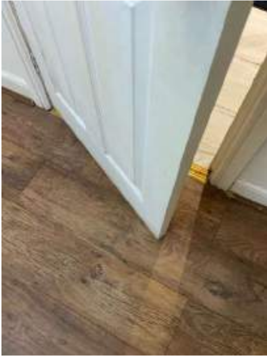
Door catches on the floor
