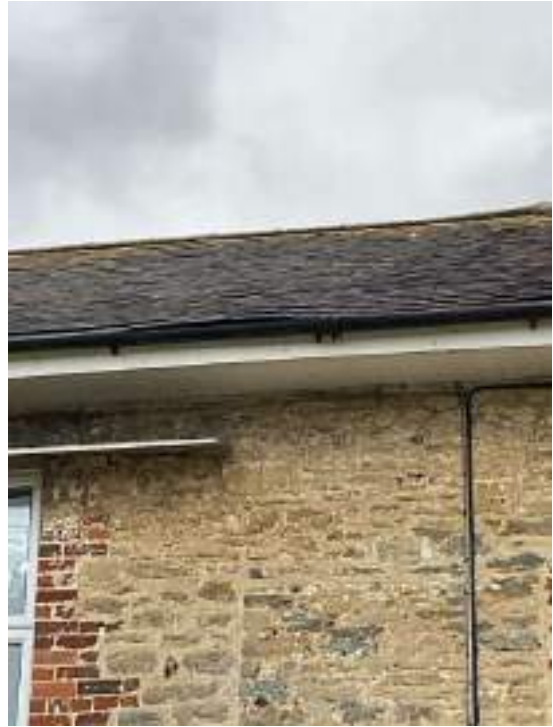
Lifted section of slates
