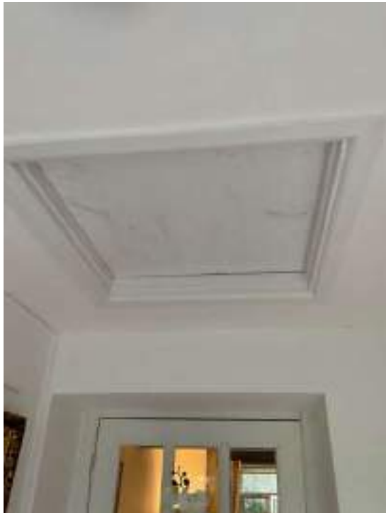
2nd hatch to ground floor roof void with cables and pipe works
