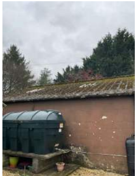
Possible asbestos containing material
