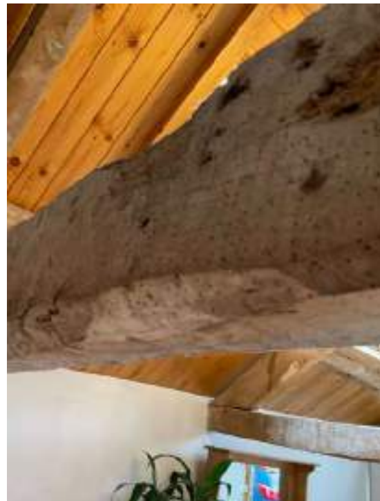
old wood boring infestation - not active
