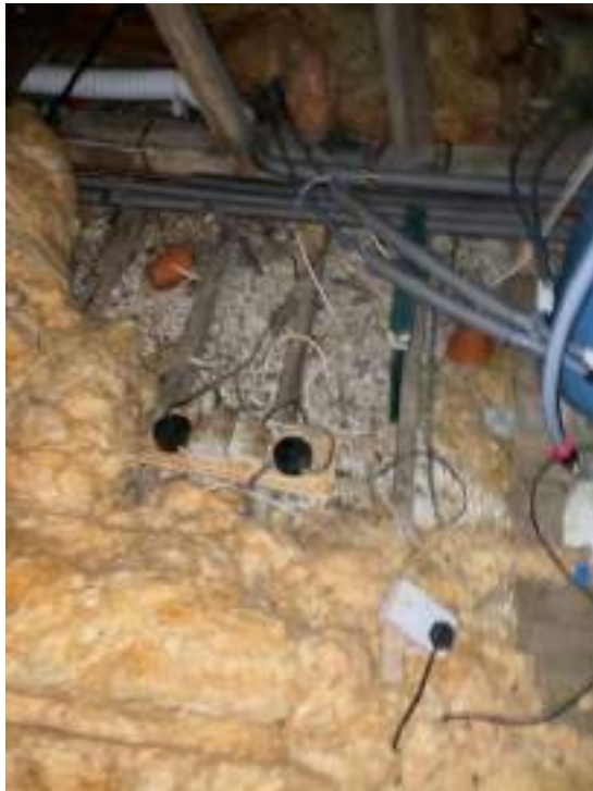
Electrics to the loft need covered
