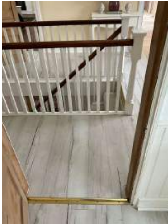
Slight spring and deflections to the first floor
