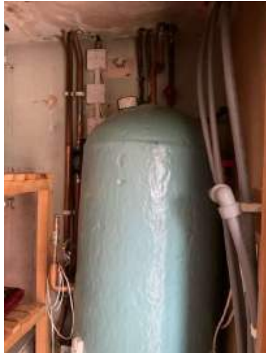
Hot water tank
