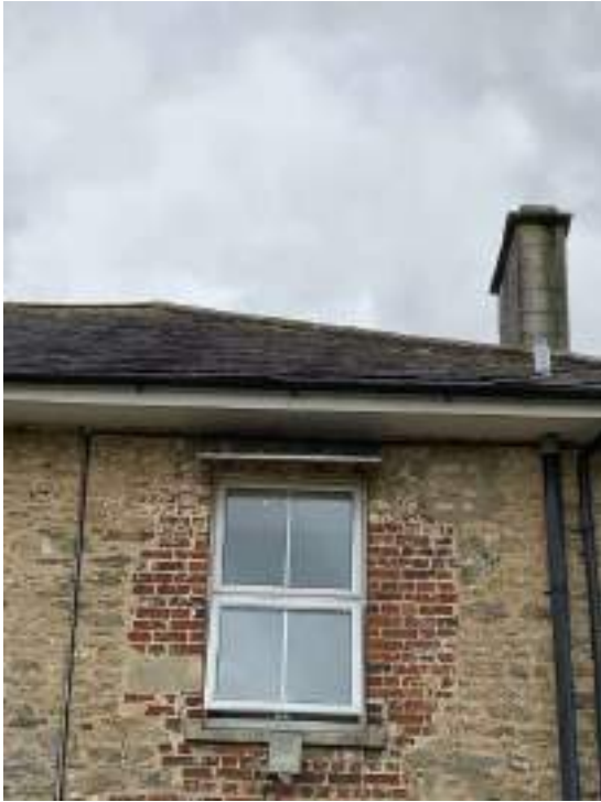
Consult a roofing contractor for costs to repair this section to the rear
