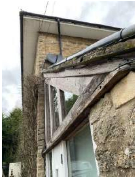
Undercloak board Possible asbestos containing material
