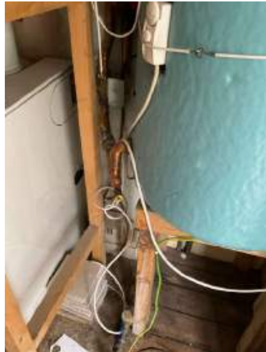
Hot water tank
