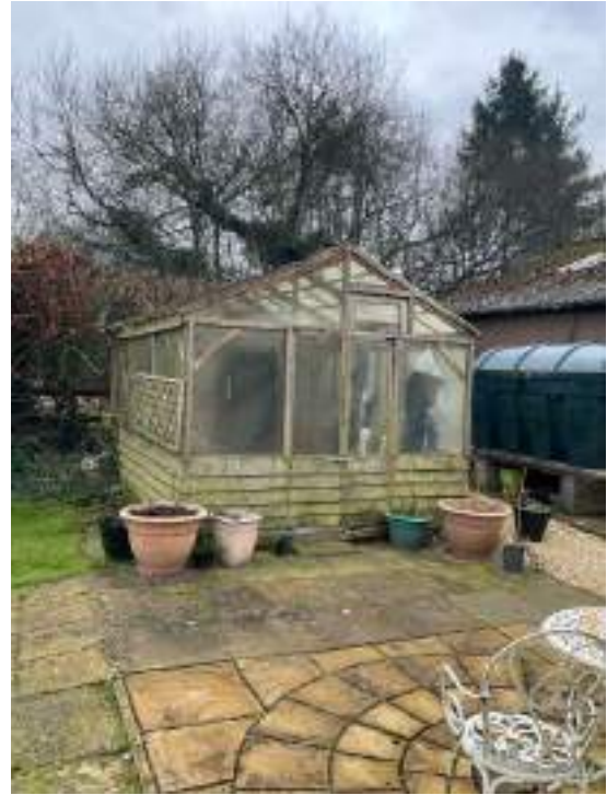
Conservatory in poor condition
