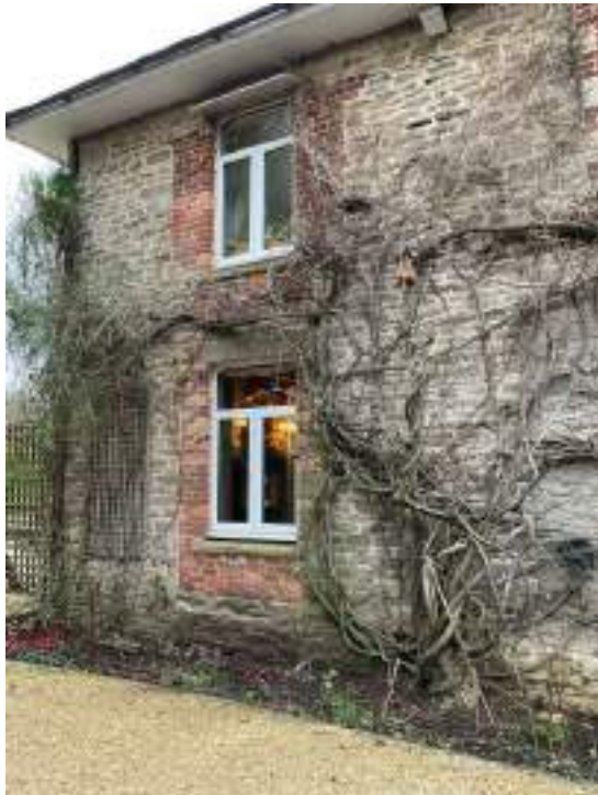
Vegetation should be removed from the walls as they soak in moisture and cause damage to the building
