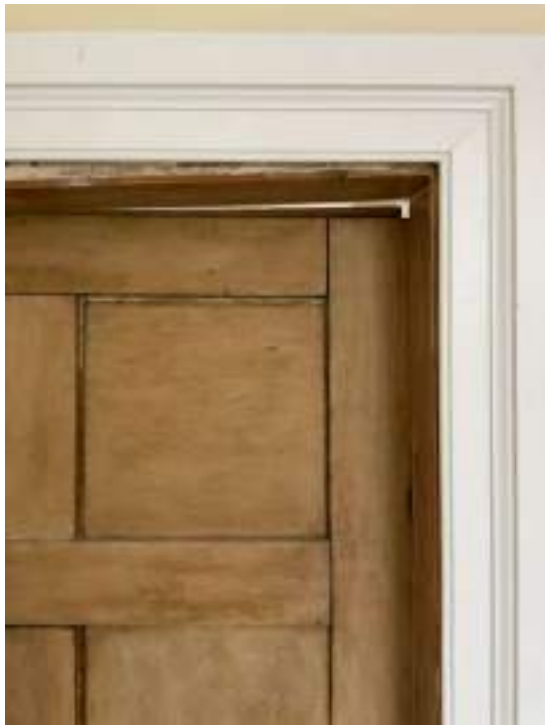
Some doors are not close fitting
