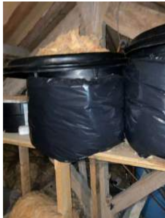
Loose fitting lids need to be replaced
