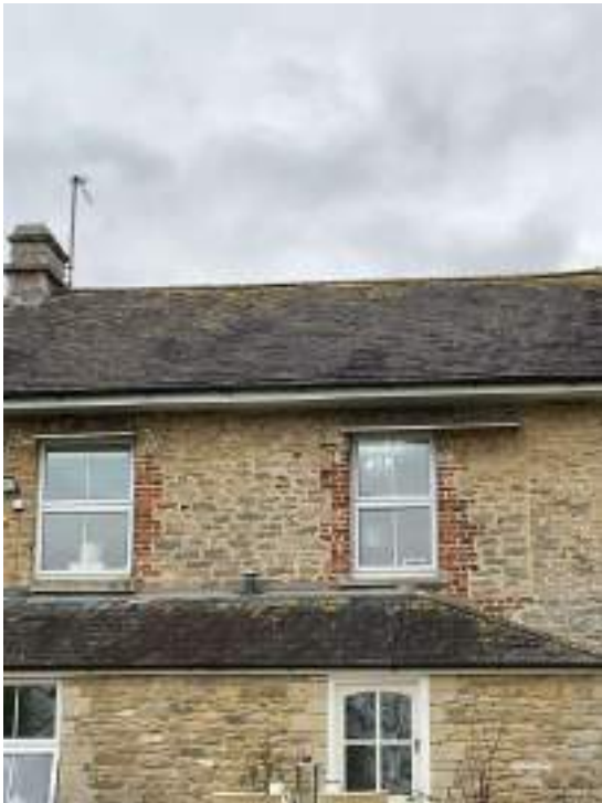
The bottom course of [redacted] have lifted which suggests the timber battens underneath have failed
