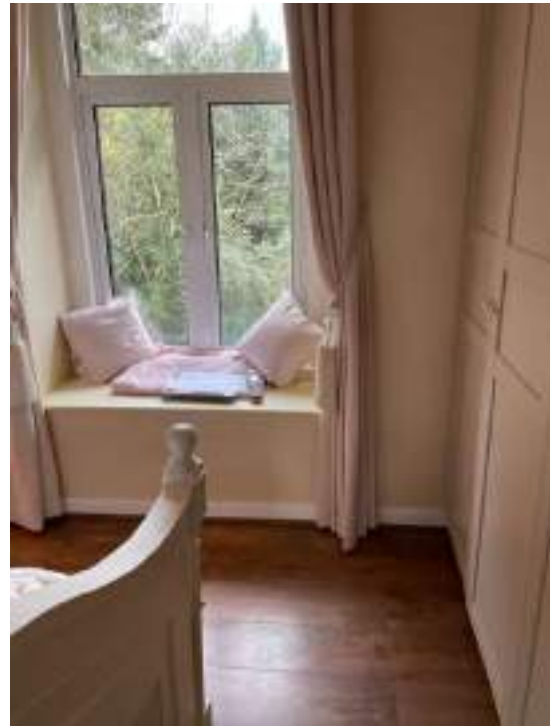
Areas of higher readings to master bedroom walls around the window
