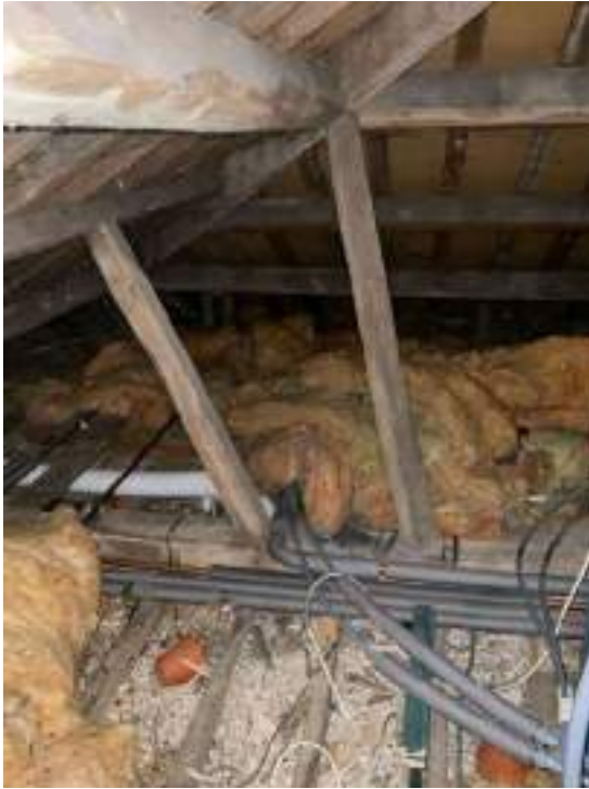
Insulated pipes, areas left un-insulated can cause cold bridging
