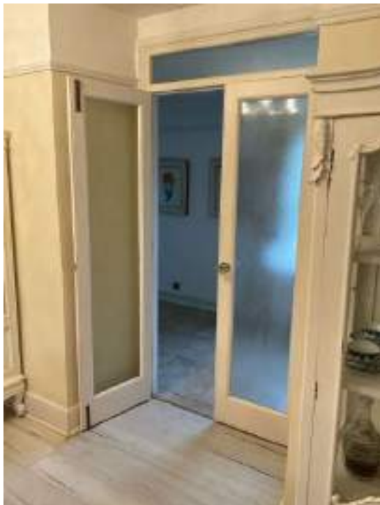
Stiff doors and no safety glazing stamps to internal doors
