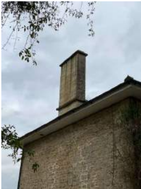
Kitchen stack condition
