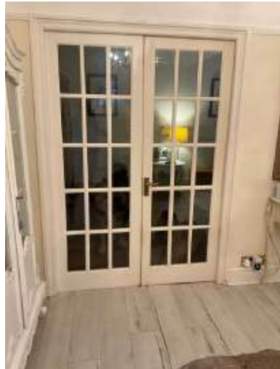
Stiff doors and no safety glazing stamps to internal doors
