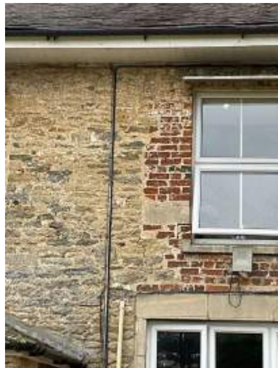
Minor cracks noted in places re-pointing required
