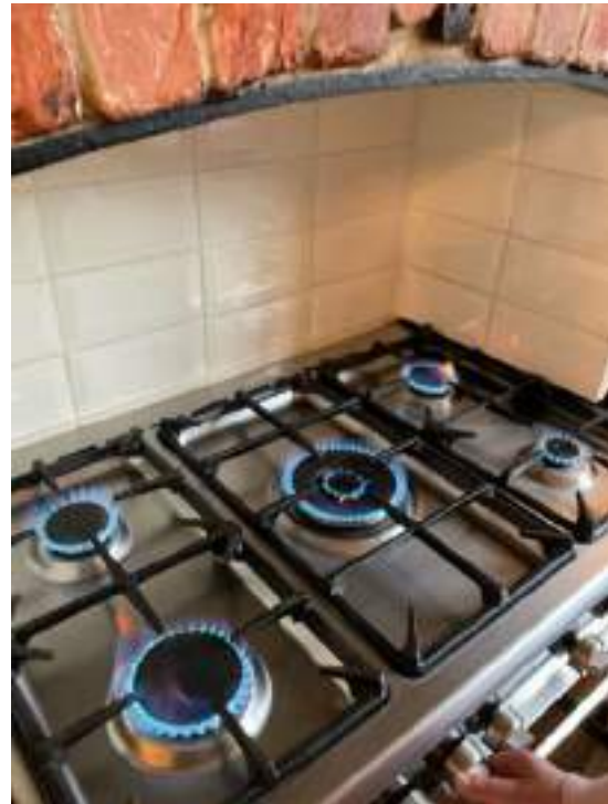
Oven and hobs tested use gas tanks
