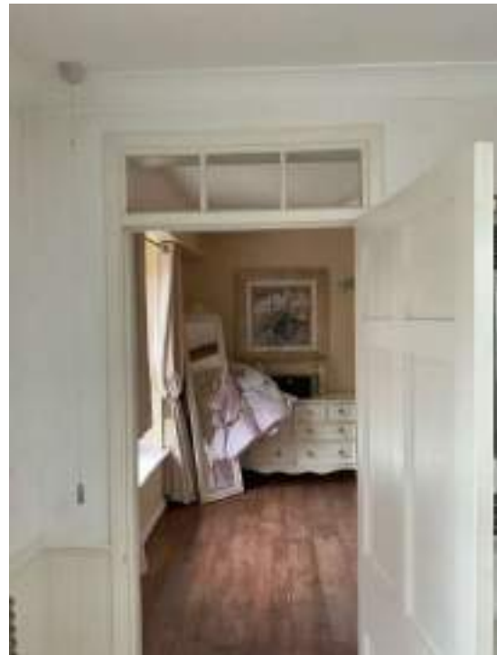
Not safe glazing
