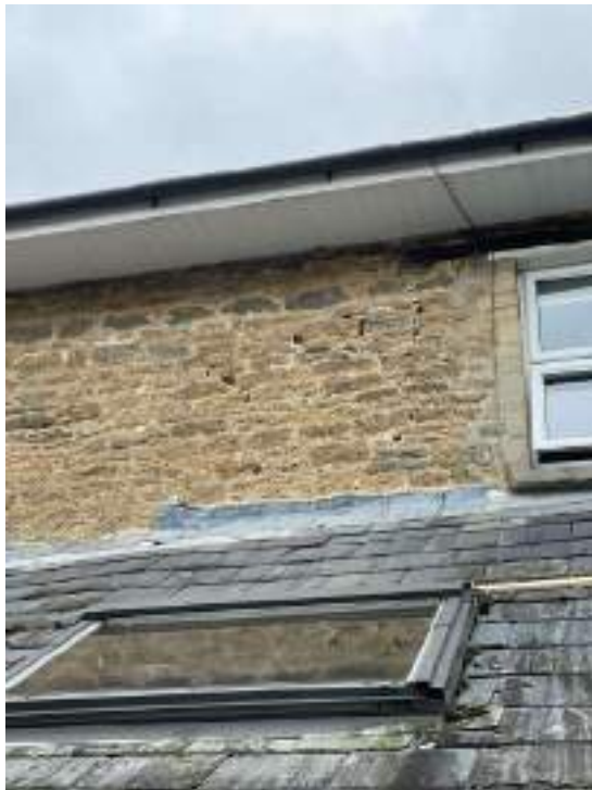
Side elevation will need re-pointed now
