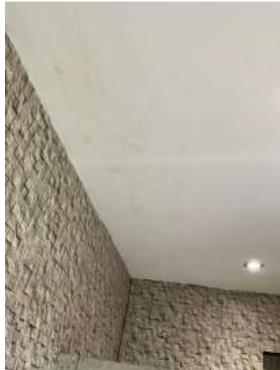
Minor re-decoration required
