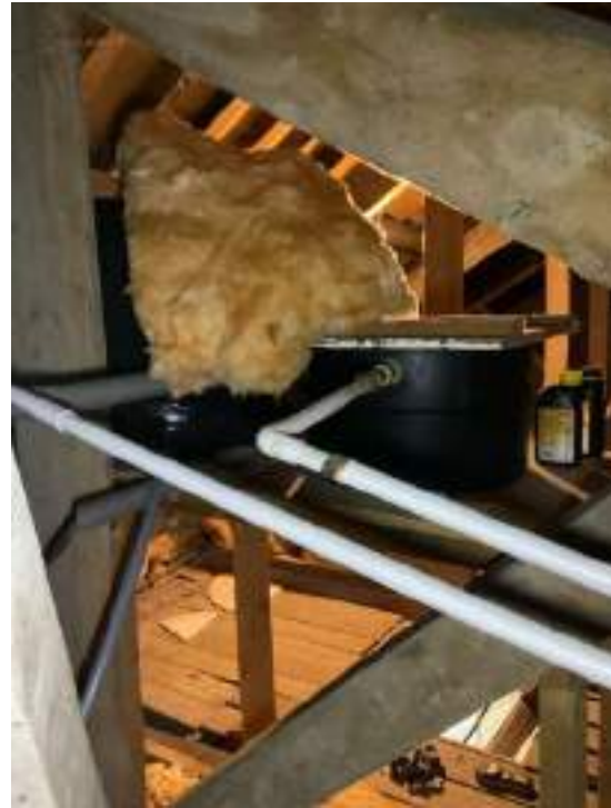
Water tanks in loft void
