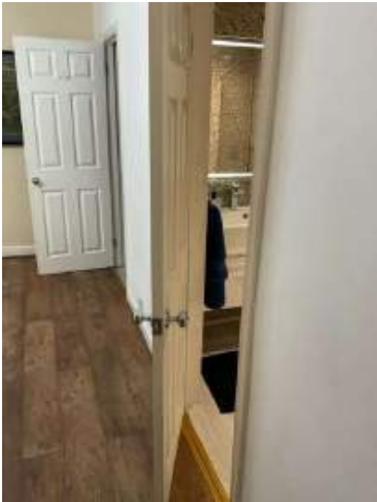
Due to timber expansion the bathroom door rubs on the floor
