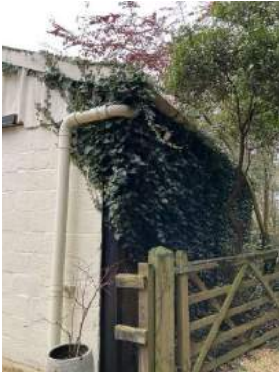
Vegetation growing out of the gutter front and rear
