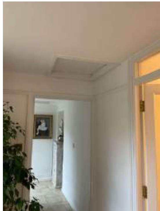
3rd hatch to ground floor
