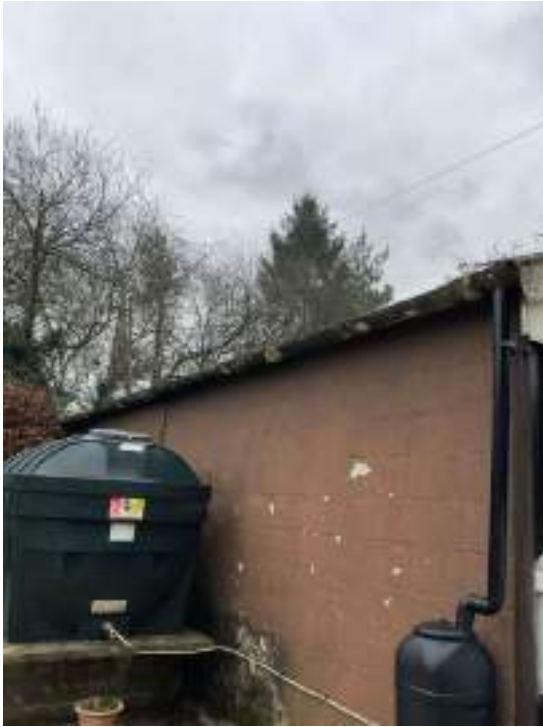
Possible asbestos containing material
