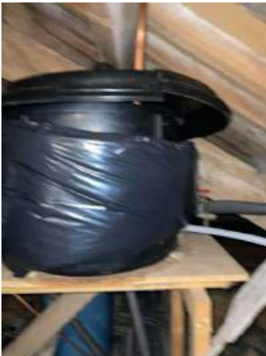
Loose covers - these need to be secure
