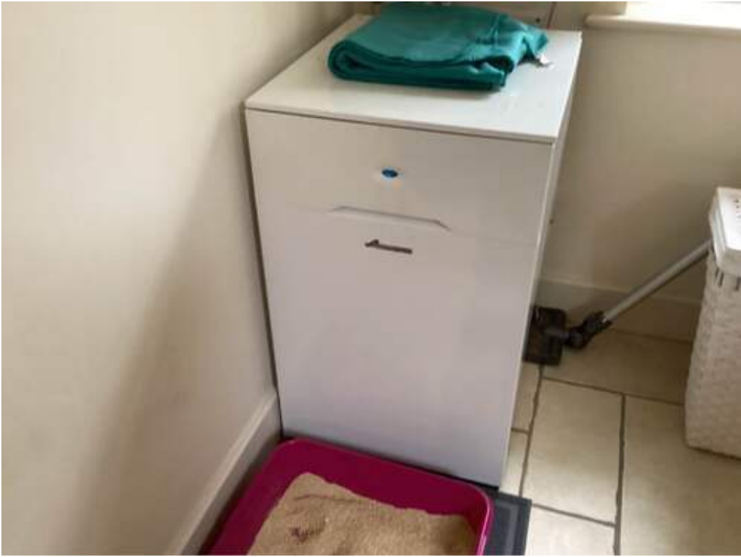
Oil fired boiler
